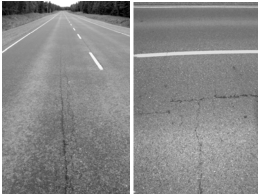
Figure 3. Spring 2006 Wheel Path Cracking in Section 3 (left) and Transverse Crack Initiation in Section 4 (right)
