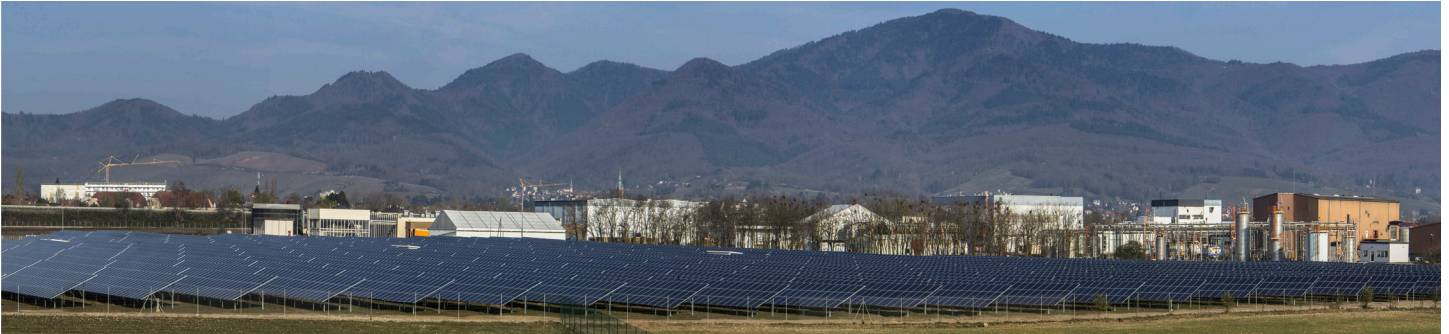
DuPont Cernay 4.5 megawatt solar park—the largest on DuPont land to-date
