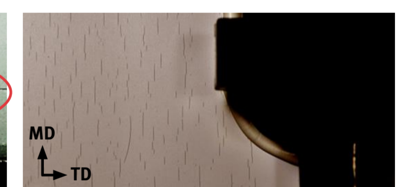
PVDF backsheet shows cracking in sequential accelerated test after one thermal cycle.
