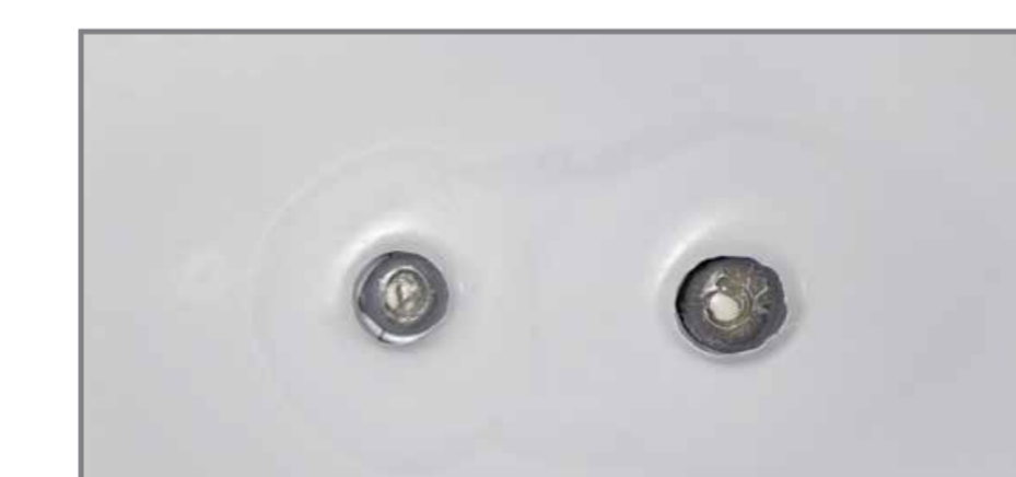
Bubbling leads to cracking
