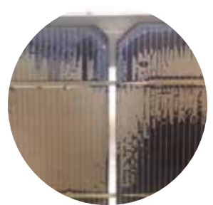
Delamination 20+ years, Italy
