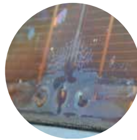
Delamination and corrosion 15 years, Southern China
