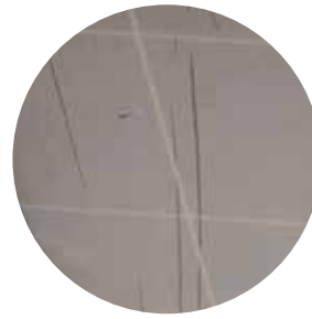
Outer-layer cracks 7 years, SW USA
