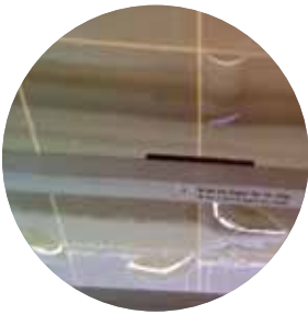
Outer -layer cracking
