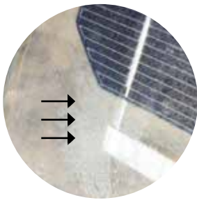
Glass/encapsulant delamination 1.5 years, Northern China
