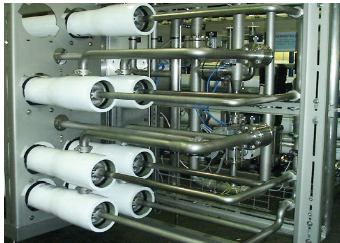
Photograph of an RO rack. Courtesy of VWS Deutschland GmbH – BERKEFELD
