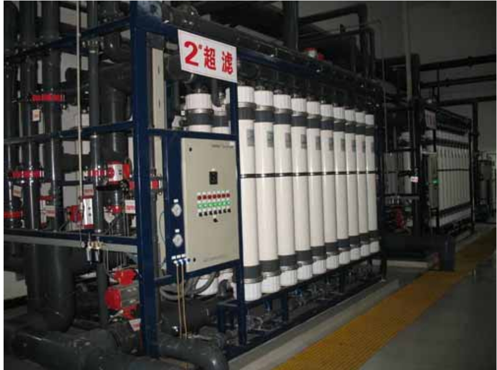
Skid 2 at the GuanYinShan cogeneration facility, using DOW™ Ultrafiltration SFP-2860 Modules. (Photo courtesy of Nantong GuanYinShan Environmental Protection Thermoelectricity Co. Ltd.)
