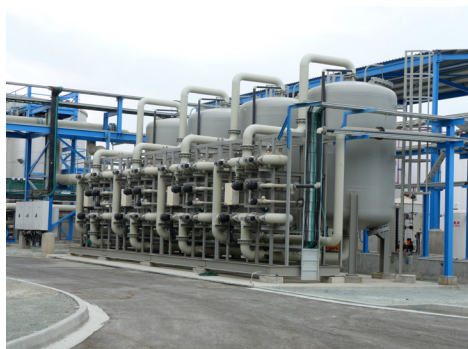
Photograph of the Boron Selective Resin system. Courtesy of MN Limassol Water Co
