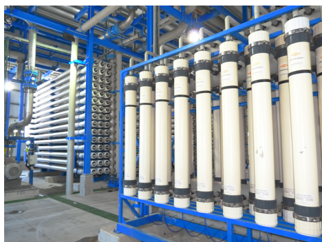
Photograph of a UF and RO train from Limassol Desalination plant. Courtesy of MN Limassol Water Co
