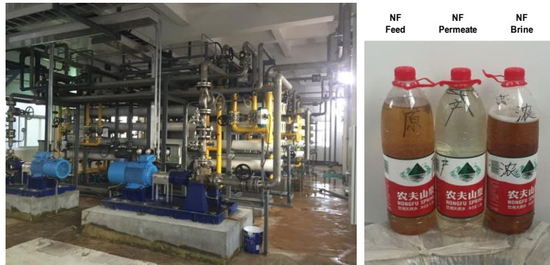
Figure 3. NF train photo of ZLD station. (Photo courtesy of SRDIPC)
