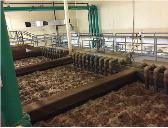
Above: The Rahr Malting Wastewater Treatment Facility was expanded and upgraded in 2008 to utilise the MEMCOR® MBR process. The membrane bioreactor plant consists of three Cells, each with 192 x B40N Modules using the MemPulse® process.
