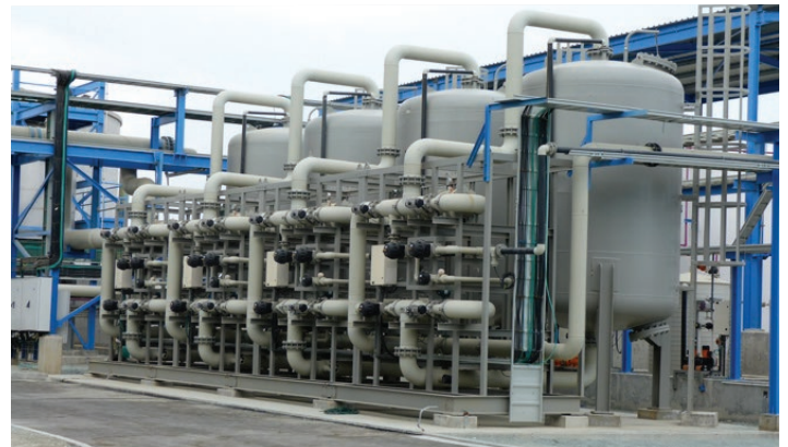
Photograph of the Boron Selective Resin system. Courtesy of MN Limassol Water Co
