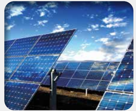
Solar PV panel
