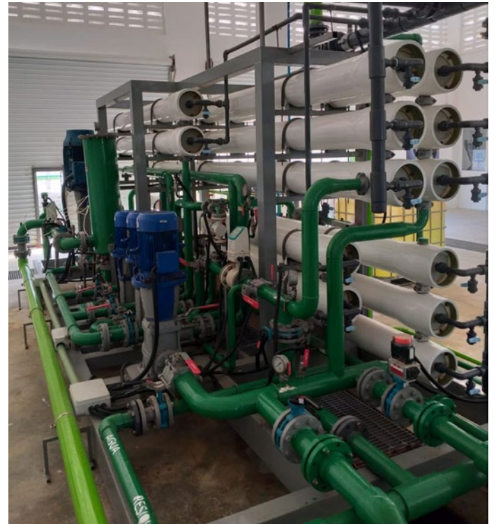
Reverse Osmosis system
